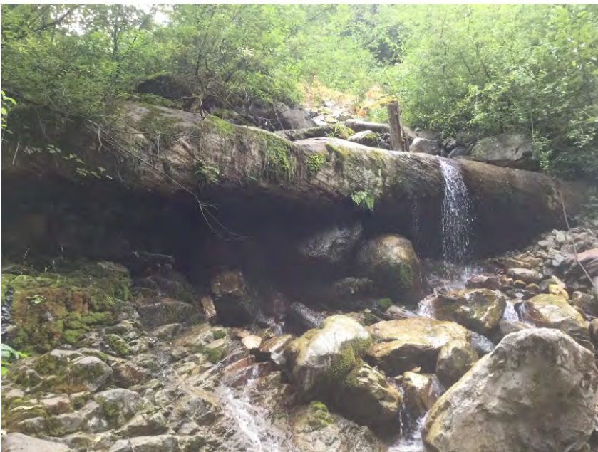
Log retaining much of the fill below culvert
